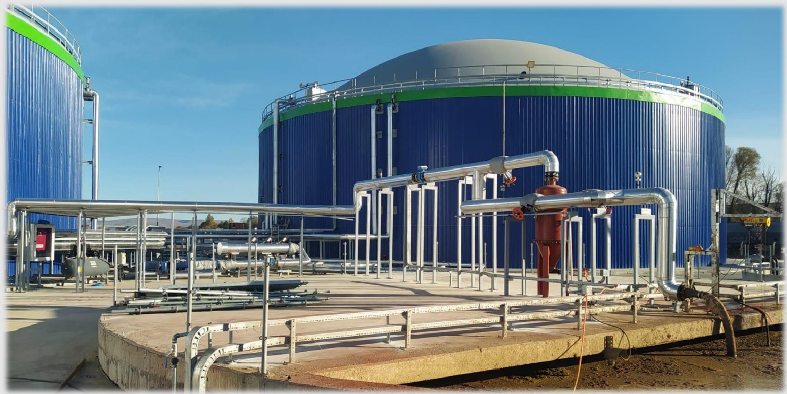
BIYOGAZ ENERJİ SANTRALİ / GAZİANTEP
